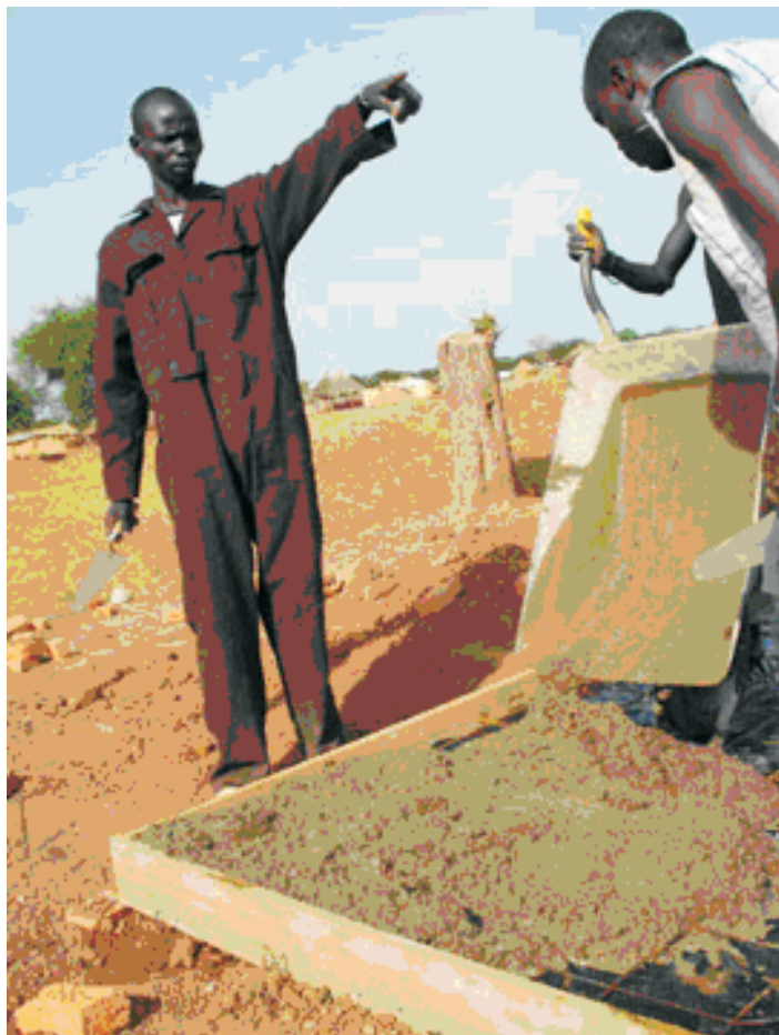
Dong Chol supervises the construction crew the Recovery and Rehabilitation Programme (RRP) has hired to build local government offices in Aweil West.
